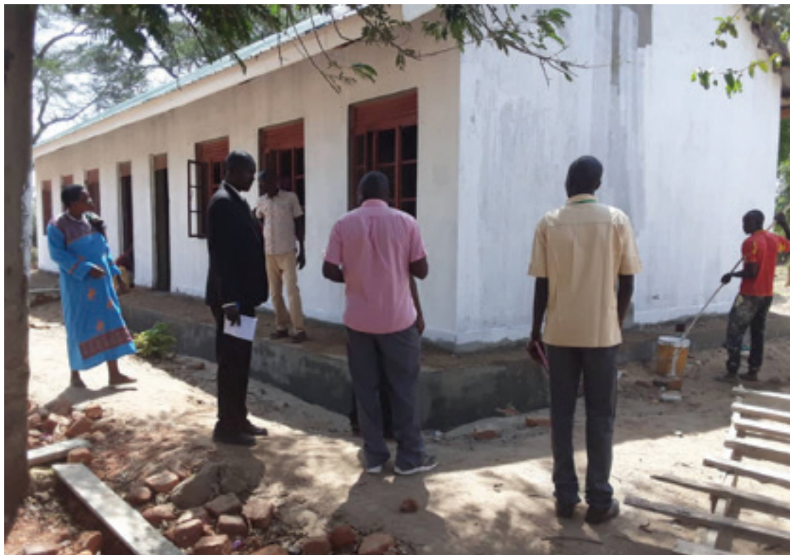
Community based monitors in Nabilatuk district inspecting construction works at Lokaala Primary School.
