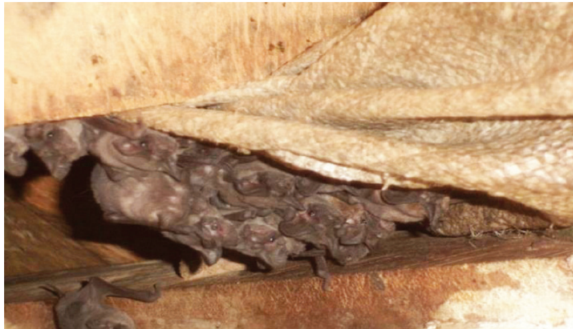
Bats occupying the roof at Abei Health Centre II.
