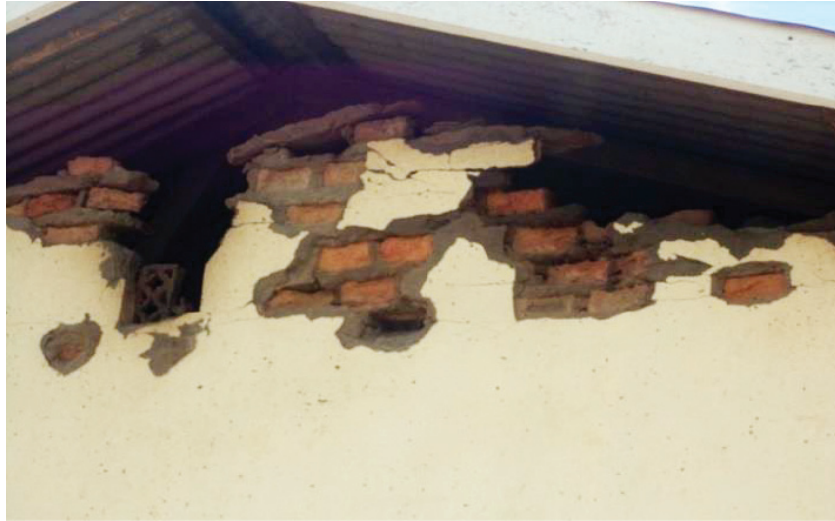
Collapsing gable ends of the OPD at Abei Health Centre II.
