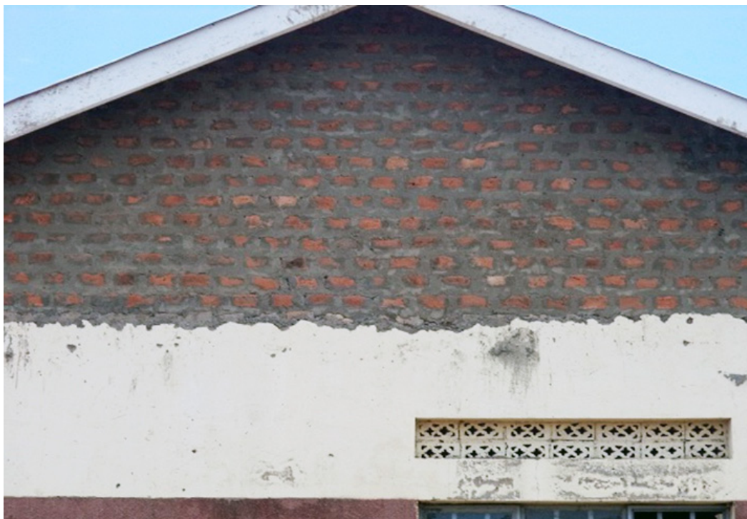
The gable ends of the OPD wall were corrected and the Health Centre was fumigated chasing away the bats.
