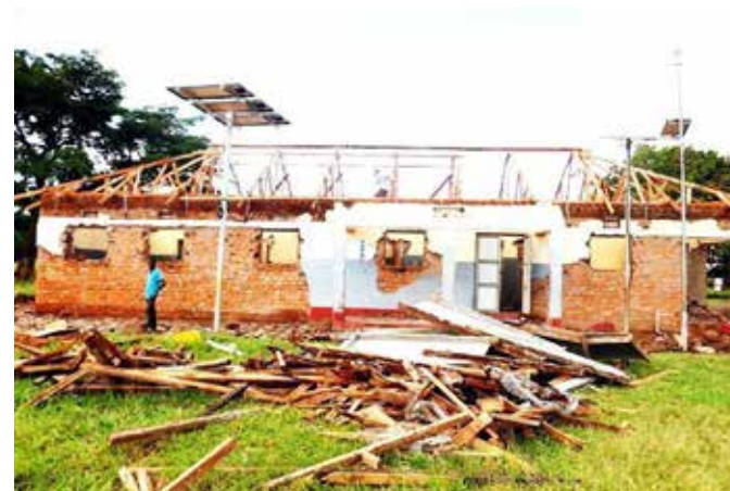
The sorry state of Chawente Health Centre III was reported to ACCU through the ICT Platform.
