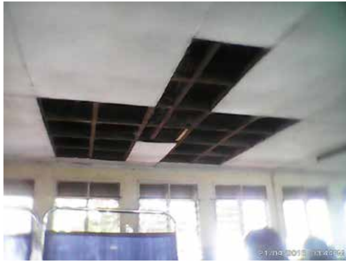
A dilapidated ceiling at Nakavule Hospital Iganga.
