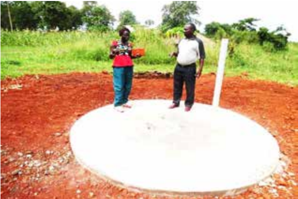
The new placenta pit constructed at Abongomola HC in Apac district as a result of a Public Accountability Forum.
